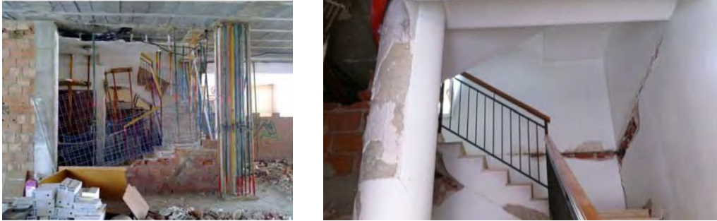
Fig. 3 – Damages to unreinforced masonry infill walls located on vertical communication cores
