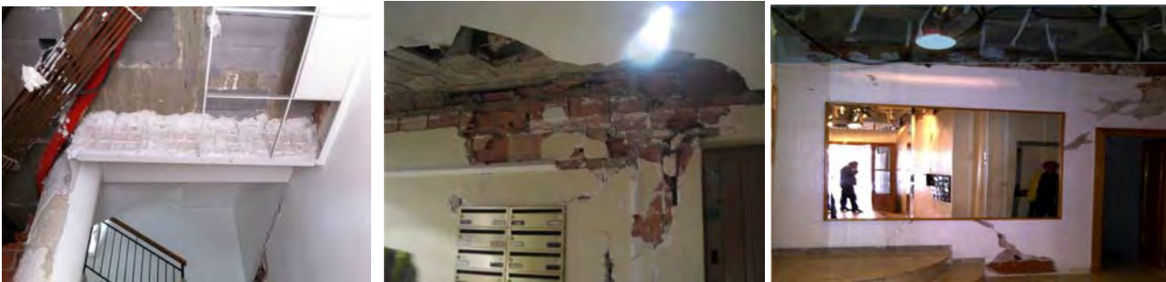
Fig. 4 – Damages to non-structural elements located in the common areas of the ground floor
