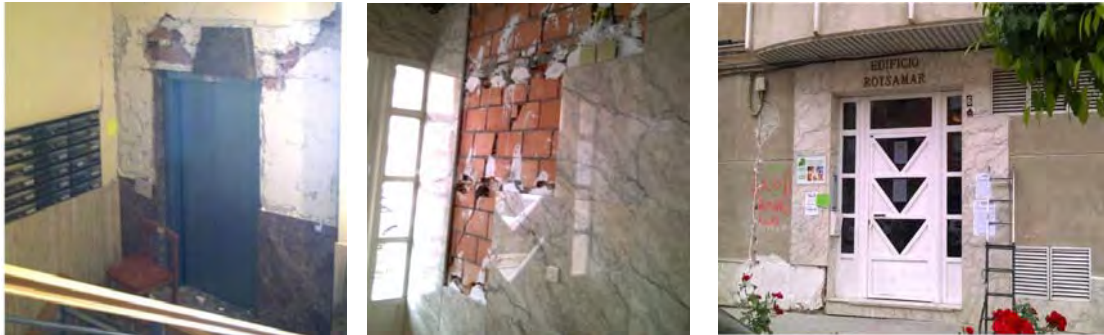
Fig. 5 – Damages to interior and exterior claddings panels
