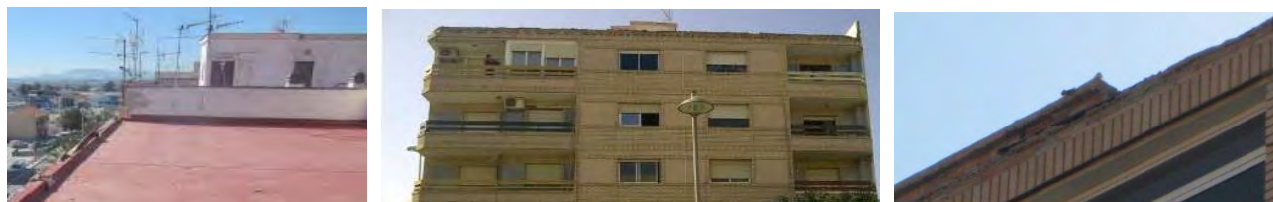
Fig. 8 – Damages to unreinforced masonry roof parapets
