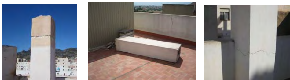
Fig. 9 – Damages to unreinforced masonry roof chimneys
