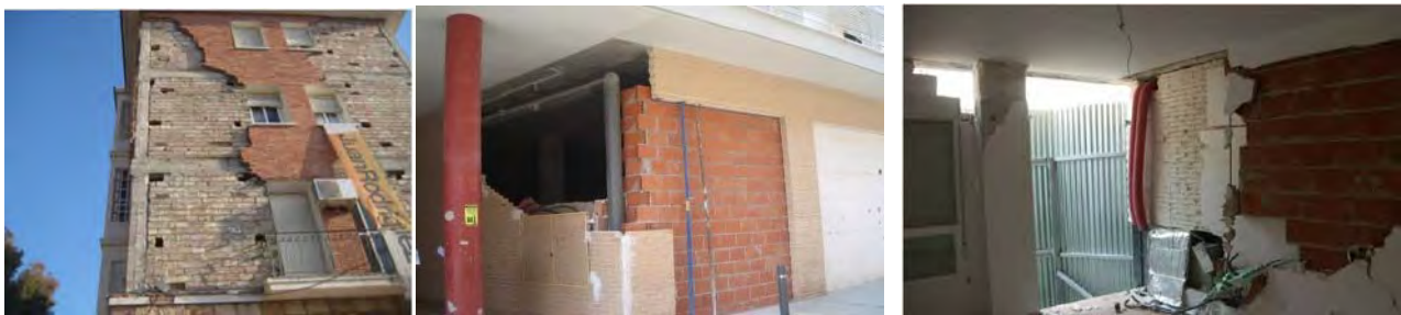
Fig. 6 – Damages to exterior infill walls (interior and exterior façades)
