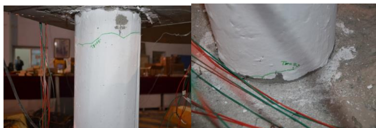
Fig.5 - circumferential fine cracks under taft wave with Y direction 0.45g
