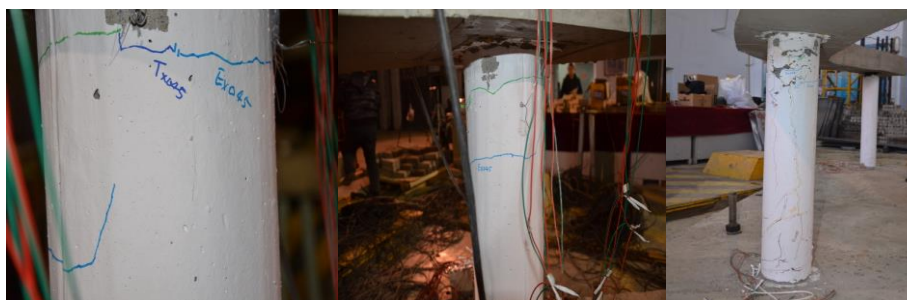
Fig.6 -Circumferential and diagonal cracks
