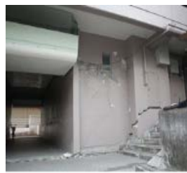
(b) Damage of base mat at the level difference
