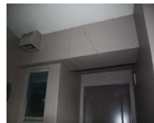
(c) Damage of a structural beam
