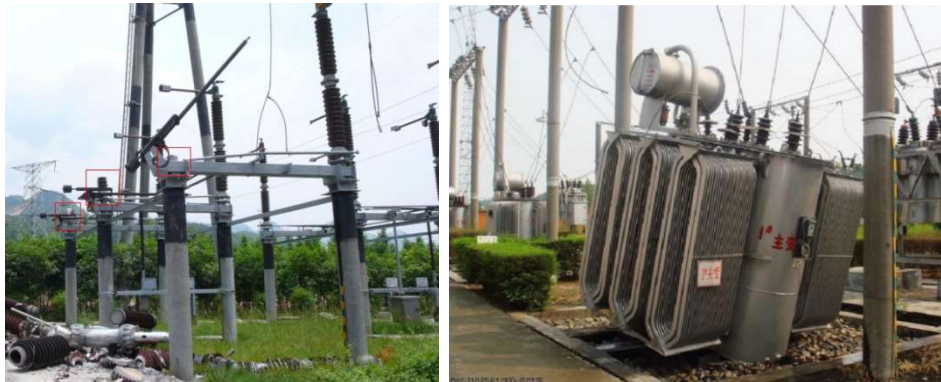
Fig. 2 Damage of cylindrical electrical equipment and transformer in 2008 Wenchuan Earthquake in China
