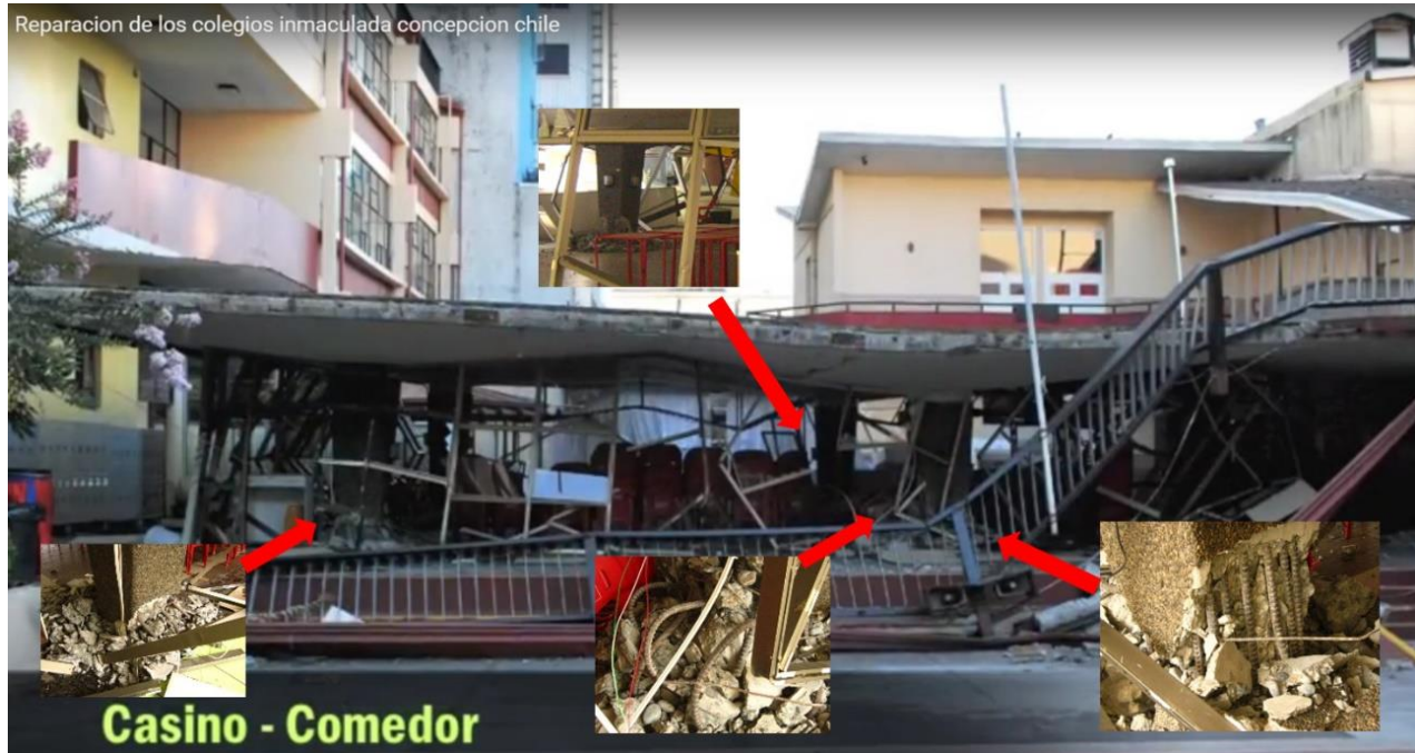
Fig. 3 - Collapsed structure and main damages. (Main photo taken from video https://www.youtube.com/watch?v=QzJFbhYWmbw . Small photographs Salvador Sáez)
