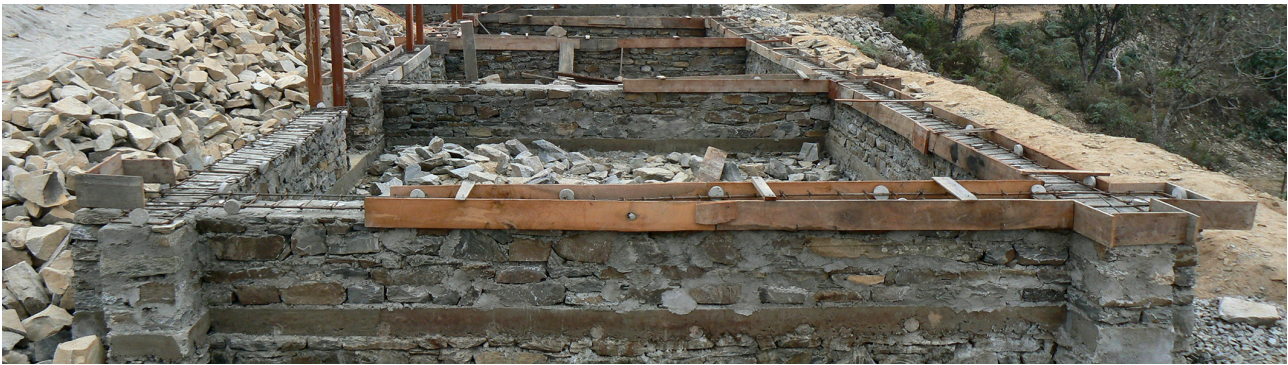
Figure 1 – Random rubble stone masonry with cement mortar, brought to courses with proper bonding, and nominally reinforced with concrete bands (by courtesy of Smart Shelter Foundation).
