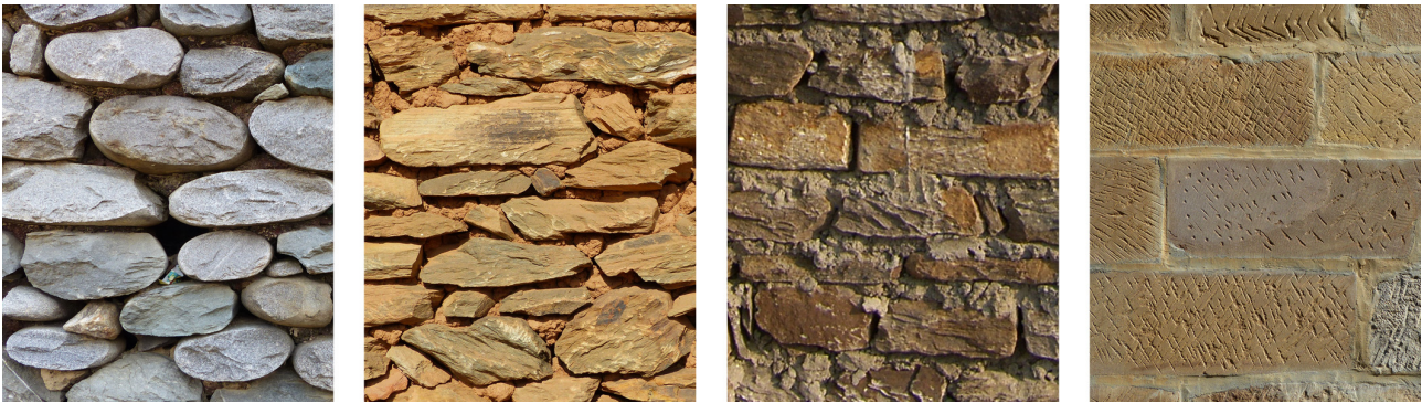
Figure 2 – a) Round river boulders with mud mortar; b) Random rubble stone masonry with mud mortar; c) Random rubble stone masonry brought to courses with cement mortar; d) Ashlar stone masonry with lime-sand mortar (all by courtesy of Smart Shelter Foundation).
