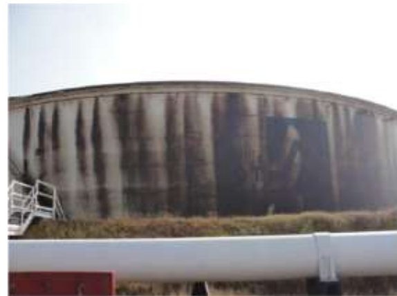
Fig. 6 - Tank T-6020 with oil spill by insufficient freeboard. ENAP Bío Bío refinery. The Maule 2010 [14].
