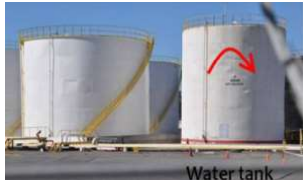
Fig. 12 - Tank with inclination perpendicular to the coastal edge. San Vicente Port, El Maule 2010 earthquake.
