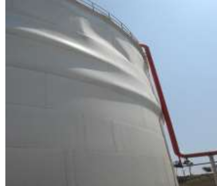
Fig. 18 – Tank for acid storage in Mejillones. Lower buckling of shell. Tocopilla earthquake in 2007.
