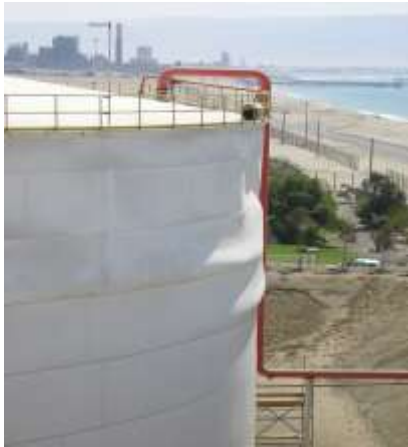
Fig. 9 - Tank located in Mejillones during the Tocopilla 2007 earthquake, buckling in the shell perpendicular to the coast.
