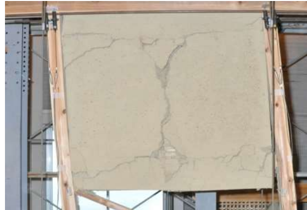
(b) Shear failure (MWD-T1500)
