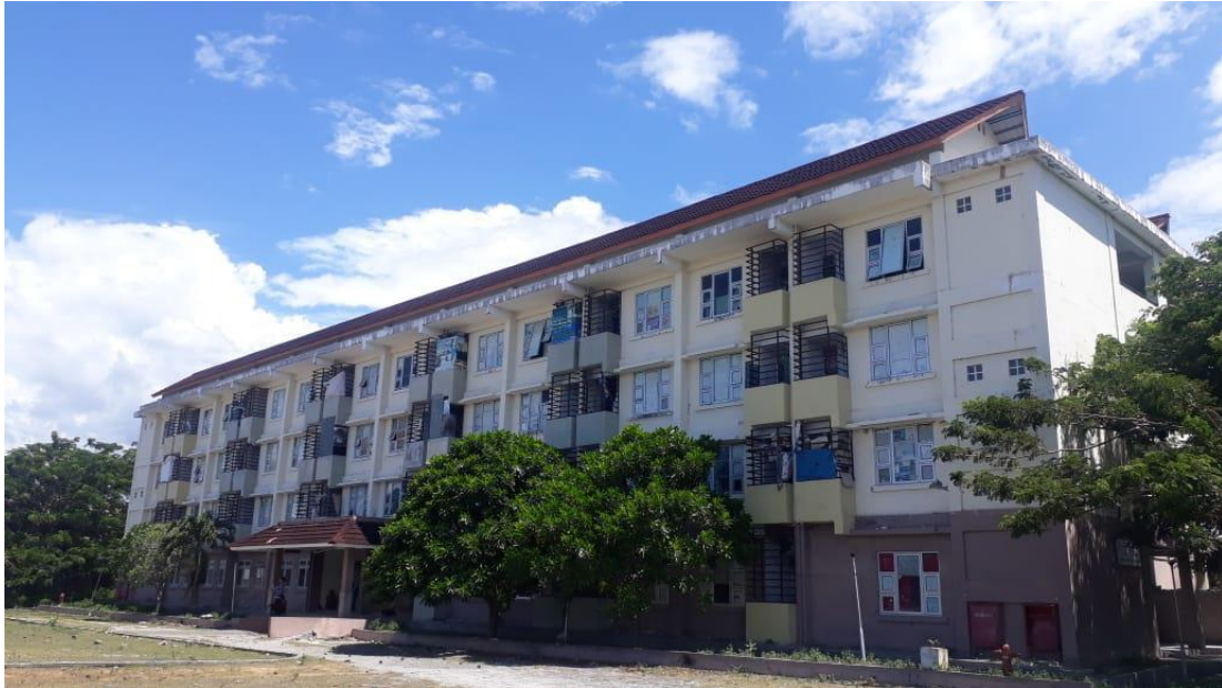
Fig. 2 – Front view of damage occurred on rental low-cost housing flat UPT Dinas PU Palu
