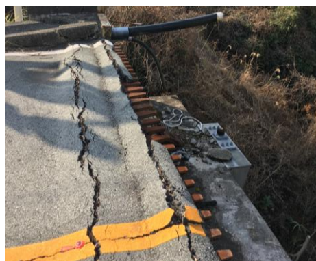
Fig. 9 – Collision or compression of explosion joint at east side abutment
