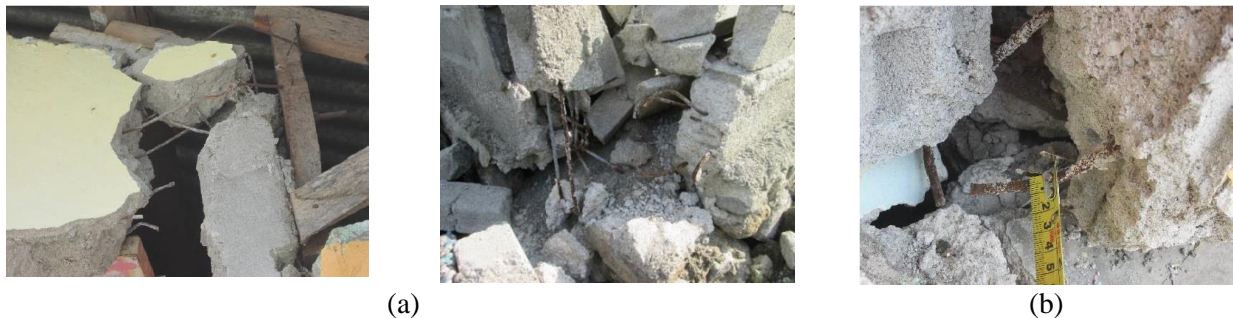
Fig. 5 – (a) poor seismic detailing and (b) poor concrete quality
