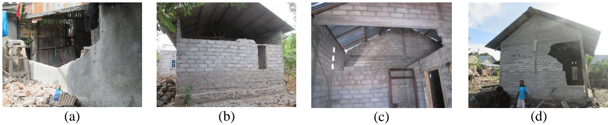
Fig. 10 – Out-of-plane collapse of wall
