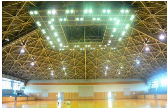
Photo 4– Hyperbolic paraboloidal steel framed shell in Chiba Prefecture (The Inside of the Same structure of Photo 3)
