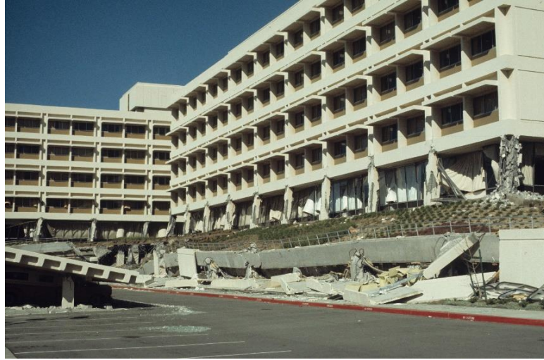
Fig. 1 – Collapse of Olive View Hospital due to presence of soft storey in 1971 San Fernando earthquake [1].
