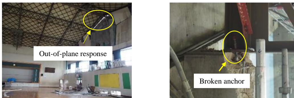
Fig. 1 Observed damage of steel roof gymnasium
