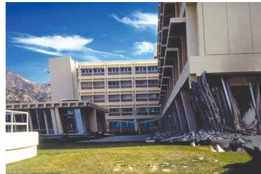
(b) Heavy damage to columns at the bottom storey
