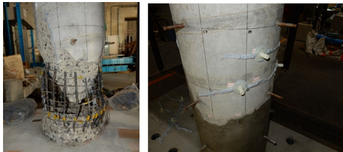
Photo 1- Repaired specimen of damaged pile
