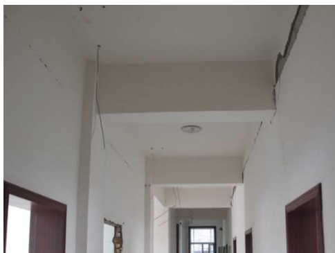
b) Loose wall under the beam
