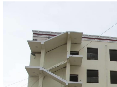
c) Wall damage
