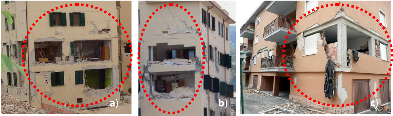
Fig. 2. Collapse of unreinforced masonry facades of multi-story R/C buildings in L'Aquila, Italy (2009).
