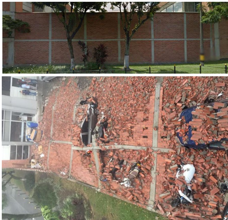
Fig. 2. – Brick URM wall prior to the collapse and resulting debris pattern (below) [1, 2] Gridlines 1-6 run from right to left in both photos.
