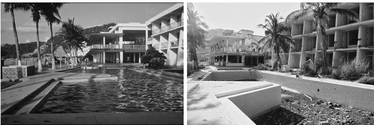
Fig. 1a (left) – Resort hotel in Barra de Navidad, México, in 1983. Fig. 1b (right) – Same hotel seen in 2003, many years after heavy damage in an October 1995 earthquake. Moment frame structure at left did not permit safe exit.
