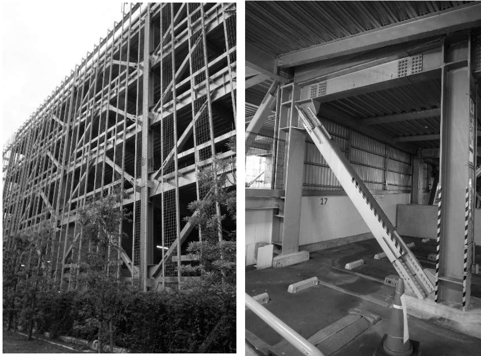
Fig. 4a (left) – Outside view of the Nagasaki Harbour Medical Center parking garage shows the extensive use of concentric braced frames. Fig. 4b (right) – Detail of one of the connections.
