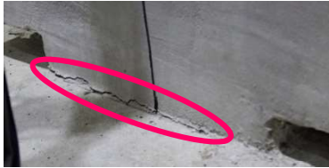
Fig.10 – Horizontal cracks on cover concrete of Mesnager hinge
