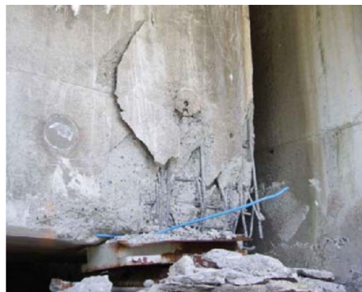
Fig. 6 – Damage of the PC box girder end supported on the A2 abutment
