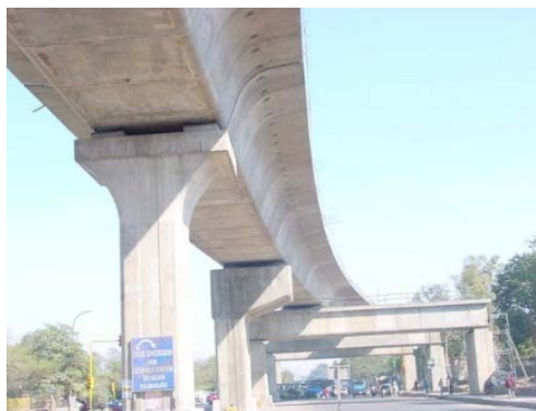
Fig. 4 – A typical configuration of eccentric C-bent pier with portal frame (Courtesy: www.tcpl.com [3])
