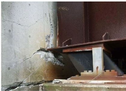
Fig.15 – Girder collided with A1 abutment
