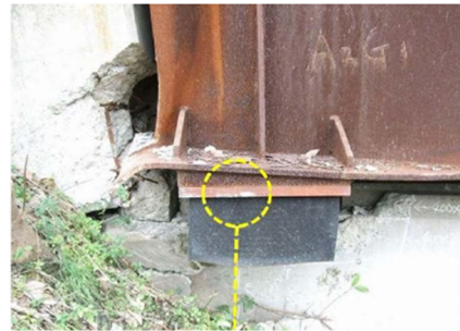
Fig.16 – Girder collided with A2 abutment
