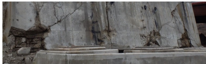
Fig.8 – Damage overview of the A2 abutment
