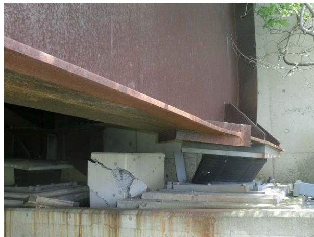
Photo 2 – Deformation of A1 support point of main girder
