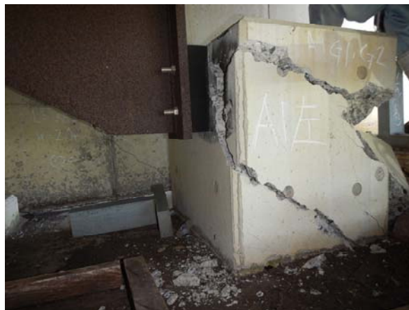
Photo 5 – Damage of the lateral displacement restraint structure on A1 abutment
