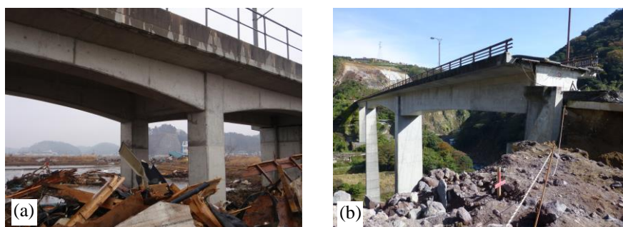
Fig. 5 – Example of resilient structures against the catastrophic event: (a) rigid frame in the tsunami affected region taken after the 2011 Great East Japan earthquake; and (b) rigid frame in the landslide affected region taken after the 2016 Kumamoto earthquake
