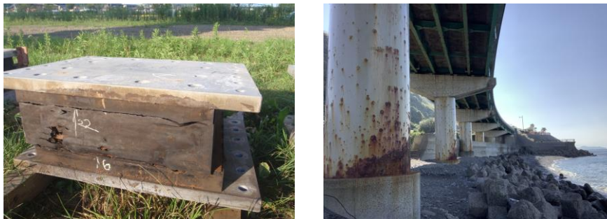
Fig. 4 – Bridge components with material deterioration
