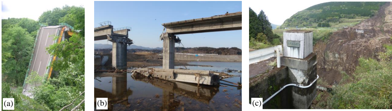
Fig. 3 – Example of bridge collapses due to the subsequent events: (a) collapse due to the land slide during the 2008 Iwate-Miyagi earthquake; (b) collapse due to the tsunami during the 2011 Great East Japan earthquake; and (c) collapse due to the land slide during the 2016 Kumamoto earthquake
