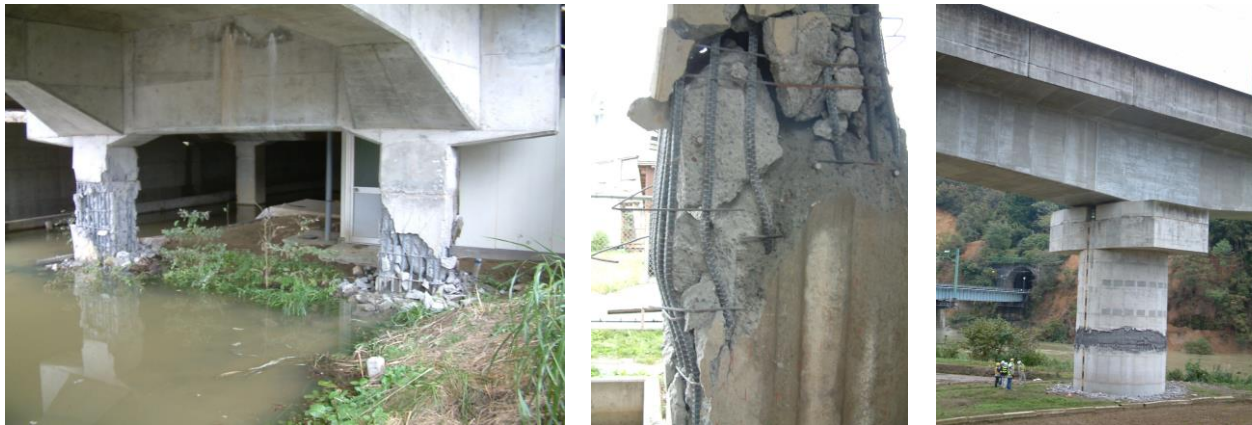
Fig. 1 – Typical failure mode of RC columns designed in the 1970s
