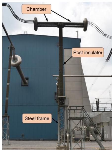
Fig. 1 –A typical high voltage bypass switch
