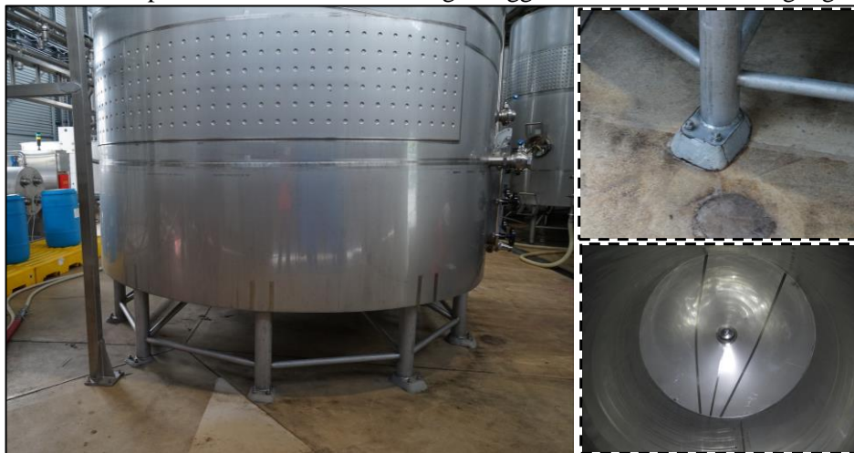
Figure 3 – An example of 50kL braced and anchored legged tank with no evidence of damage
