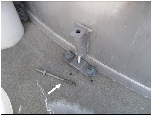
(a) Rupture of anchor rod
