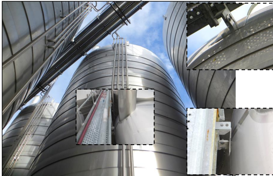
Figure 9 – An example of tank-supported catwalks with no evidence of damage following the 2016 earthquake
