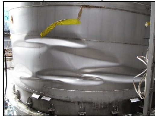
(b) Diamond-shaped buckling
