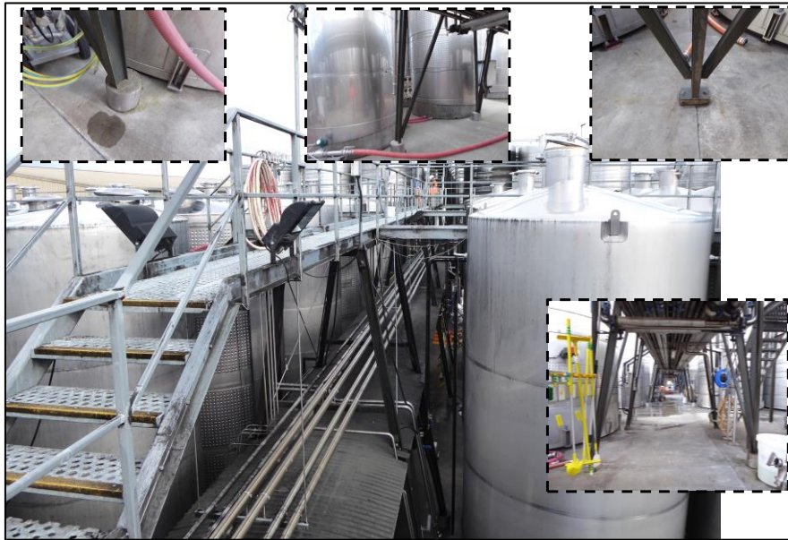
Figure 8 – An example of self-supported catwalks with no evidence of damage following the 2016 earthquake
