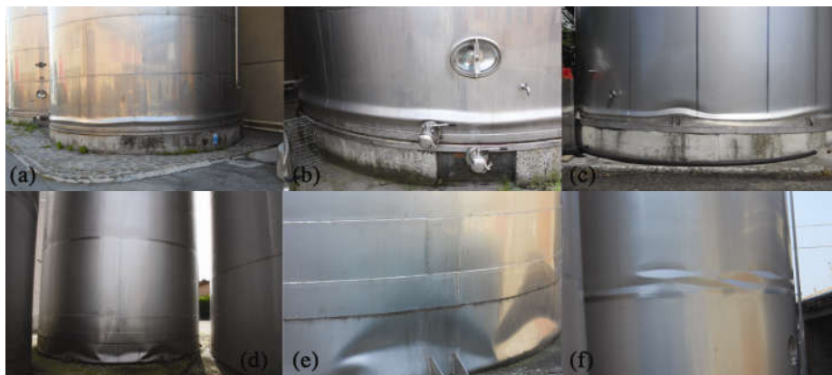
Fig. 1 - (a-c) Elephant's foot and (d-f) diamond-shaped buckling mechanisms observed in the aftermath of the May 2012 Emilia seismic sequence
