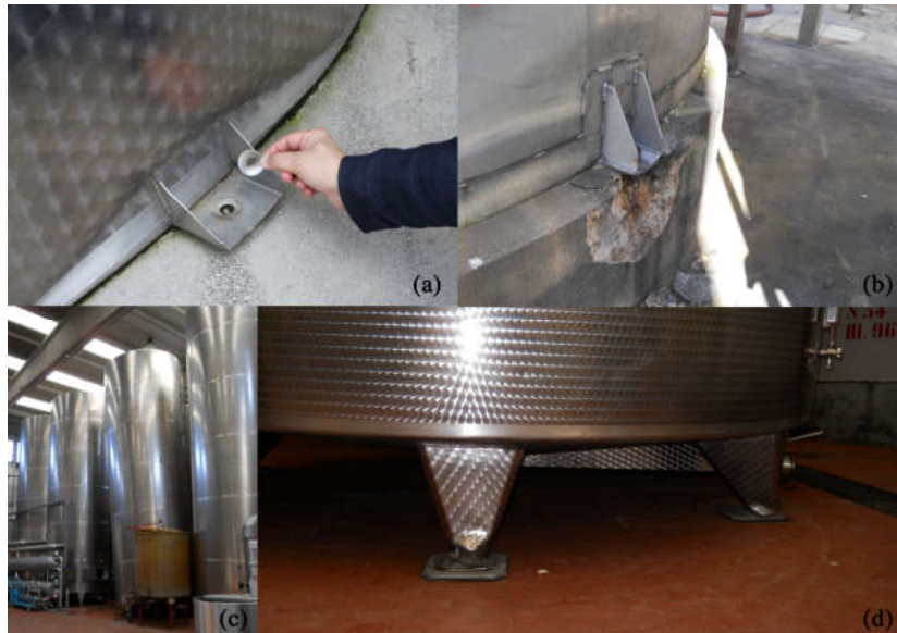
Fig. 2 - Anchoring system-related modes experienced in (a-b) flat-base and (c-d) leg-supported storage tanks during the May 2012 Emilia seismic sequence: (a) fracture of anchors and (b) concrete spalling at the anchorage; (c-d) loss of verticality due to shear-buckling in stocky tapered legs
