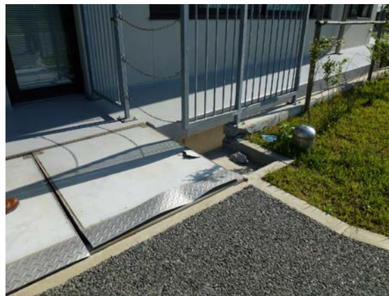
Fig. 8 A deformed gap cover
