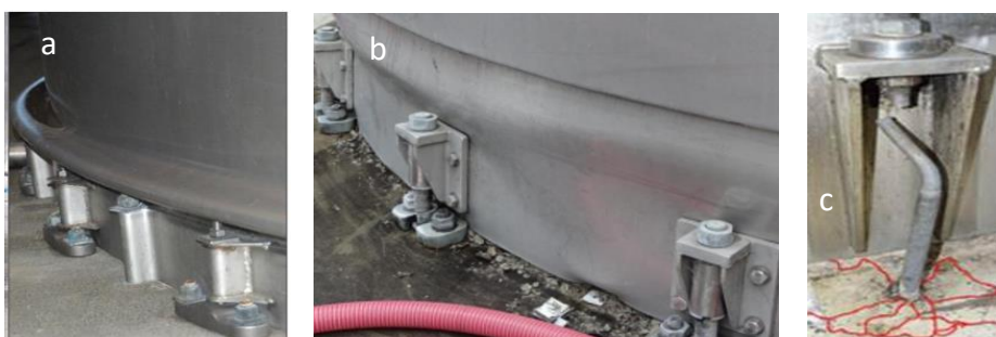
Fig. 4 – Reported damage in Kaikoura earthquake; (a, b) Barrel buckling; (c) Rod rupturing [14]
