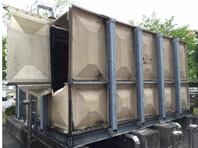
Photo 1 Example of damage to the upper of the corner and the ceiling (FRP tank) (Minami-ku, Kumamoto City)
