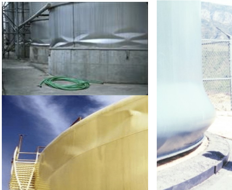
Fig. 1 – Tank's typical forms of collapse: diamond-shaped buckling (top-left), elephant-foot buckling (right) and roof damage due to sloshing (bottom-left)
