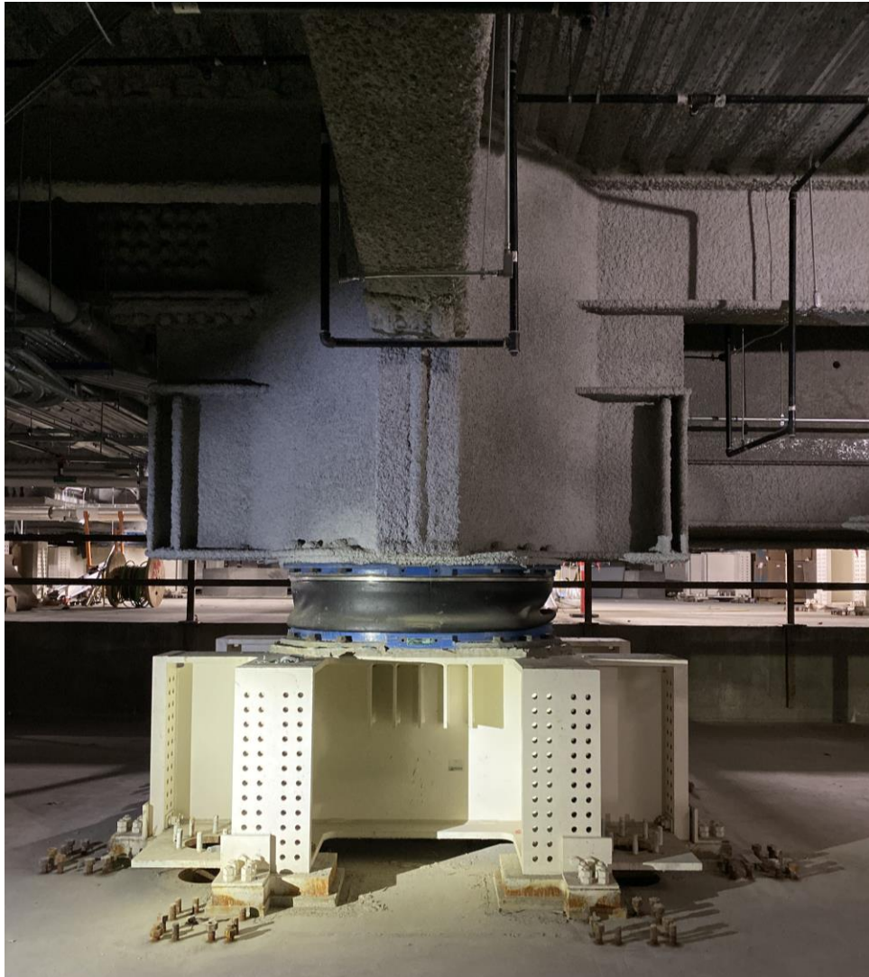
Fig. 11 – As-built condition of the VIS pedestals supported on grouted steel shims
