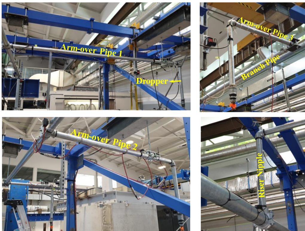
Fig. 4 – Different piping segments
