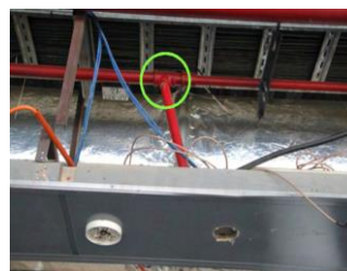
b. Fractured tee joint
