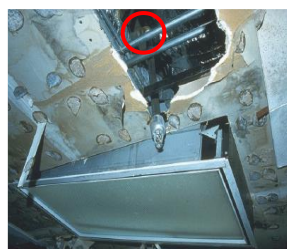
a. Fractured elbow joint
