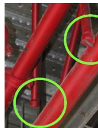
d. Damaged braces
