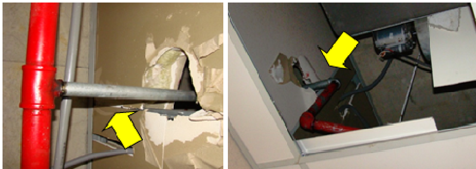
Fig. 1 – The damaged sprinkler drop in the sample hospital
