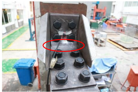
(c) Top angle ruptured at Section SA (3, \Delta = 372 mm, F = 487 kN)
