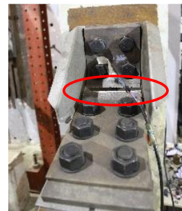
(f) Top angle ruptured at Section NA (6, \Delta = 496 mm, F = 327 kN)
