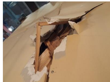
(c) Bracing damage (1/50 rad)
