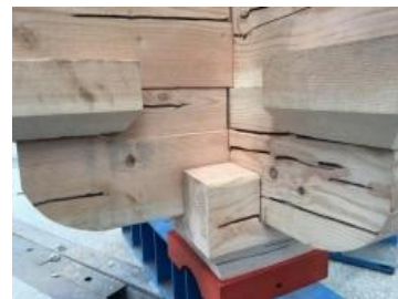
(b) Development of horizontal cracks at the bottom
