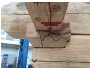
(c) Oblique cracks of the Sandou
