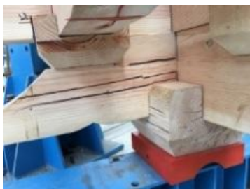
(a) Horizontal crack of the Touang
