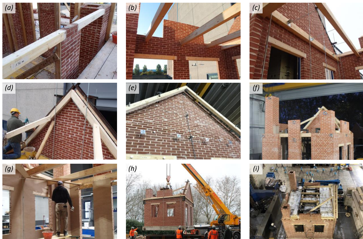
Fig. 2 – Construction details of the building specimens: (a) timber lintels at West façade; (b) floor diaphragm during construction; (c) wall-to-diaphragm connections at North façade (initially deactivated); (d) truss and struts at North gable; (e) end-plate outside the North gable (initially at distance); (f) chimneys and parapets (South-East view); (g) rendering of building interior; (h) transportation of building specimens; (i) additional masses on the floor diaphragm (top East view).
