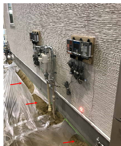
(2) Bent polyethylene gas pipes
