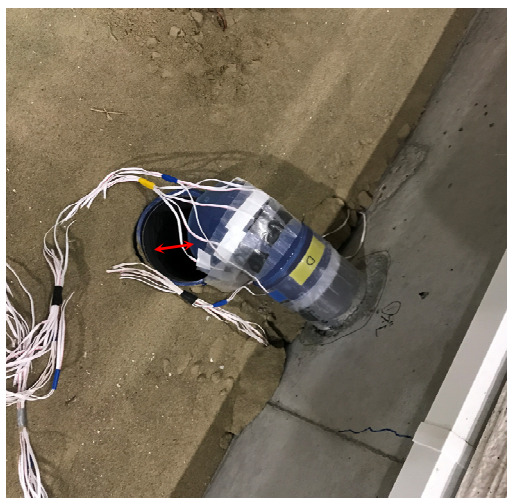
(1) Fractured VP drain pipe
