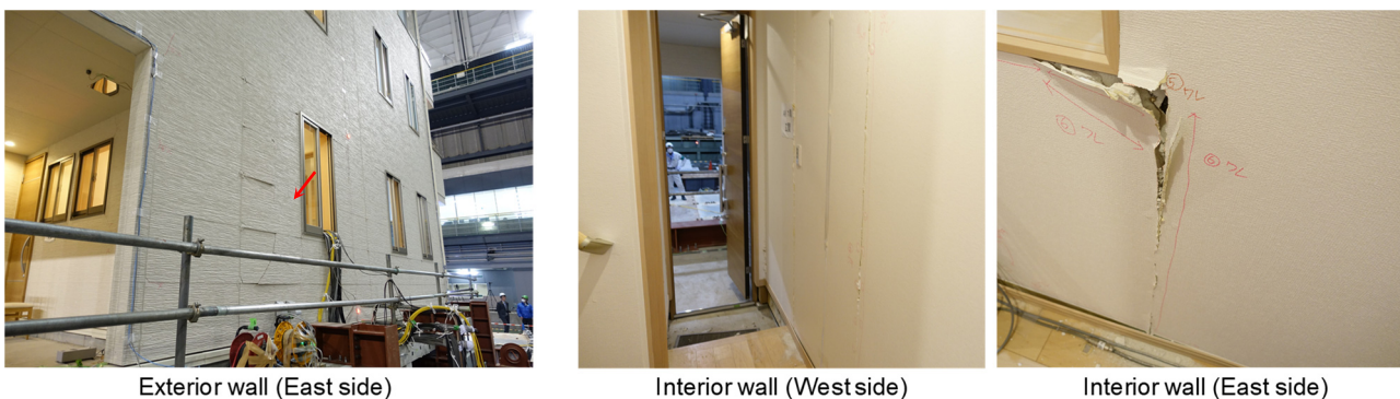
Fig. 7 Damage to the first story of A-building in the story drift of 0.03 rad (JMA-Kobe 100%)
