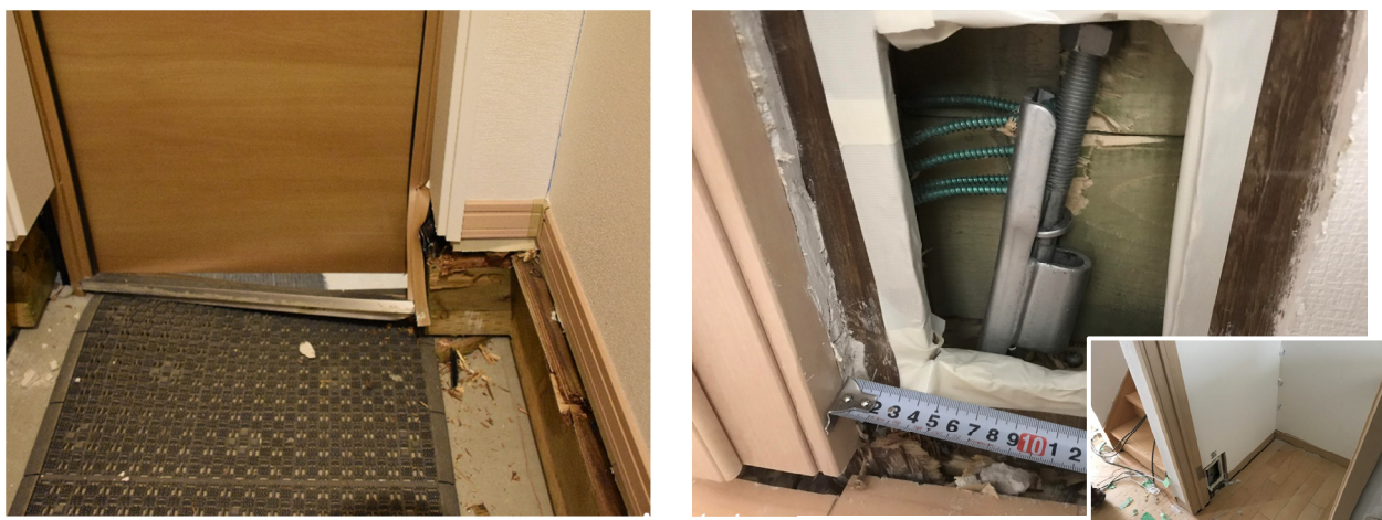
Fig. 11 Wall base fracture at the south exterior wall and screws pulled out at column base (B-building after subjected to JMA-Kobe 100%)
