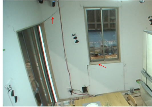
(2) Cracks slightly progressed in the interior walls under cyclic deformations
