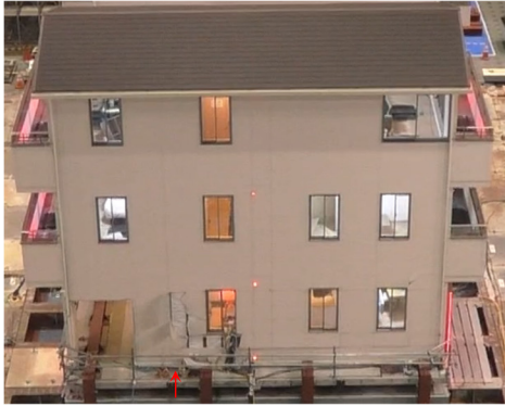
(1) Fractured and spalled siding boards came off in the cyclic drift angle of 0.04 rad
