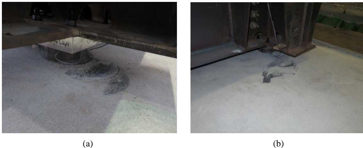
Fig. 4 –Observation of the motor base surfaces: (a) after JMA Kobe 50%_2D shaking; (b) after JMA Kobe 100%_2D shaking
