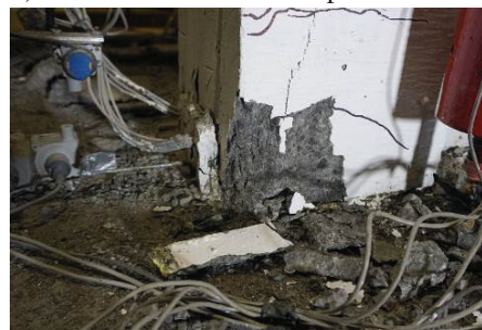
d) Extent of damage on the west side boundary element at the end of test
