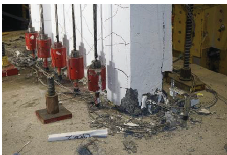
c) Extent of damage on the east side boundary element at the end of test
