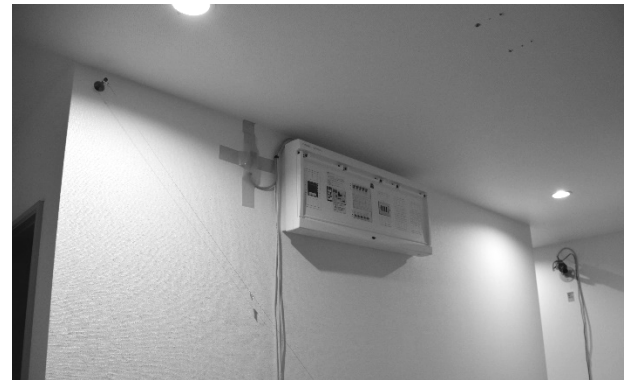
Fig. 4 – Seismic Electric Breaker of 1st story.
