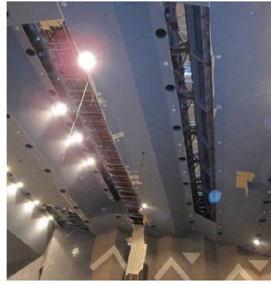
(b) – Damage to concert hall ceiling [2]
