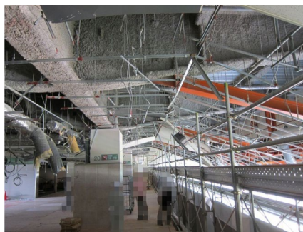
(c) – Damage to viewing hall ceiling [2]
