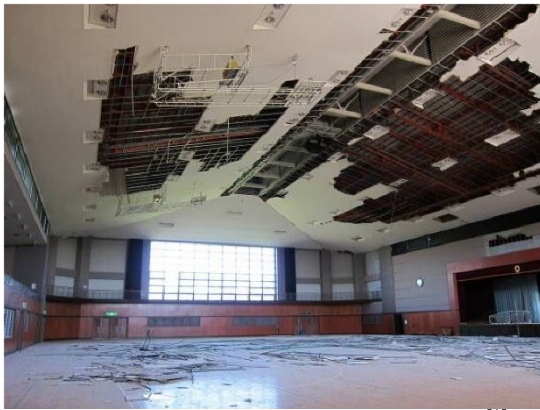
(a) – Damage to sports arena ceiling [1]
