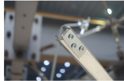
(c) Failure of brace mounting bracket
