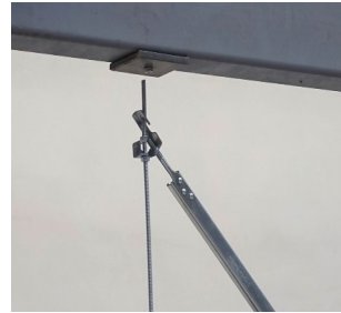
(b) Early fracture due to low cycle fatigue of suspension bolt
