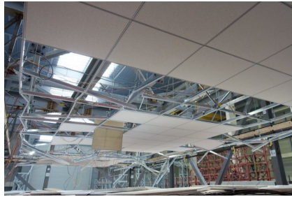
(a) The situation of the panel falling
