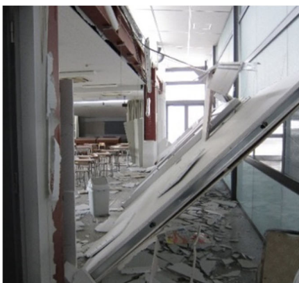
Fig. 1 – Damage of LGS wall in Kumamoto earthquake 2016
