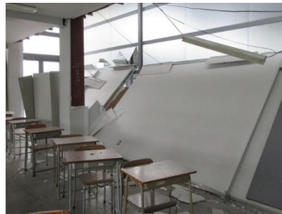
Fig.1 Damage of LGS wall in Kumamoto earthquake
