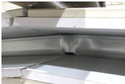
Fig.9 Local buckling of stud at the center of wall
