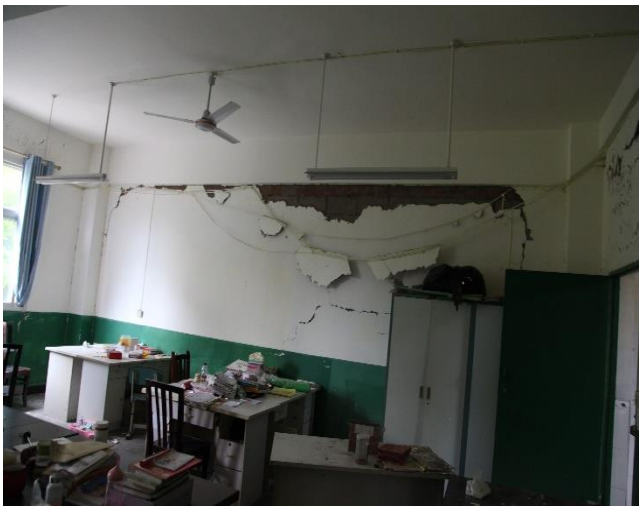
Fig.24 – Damaged masonry infill inside the building
