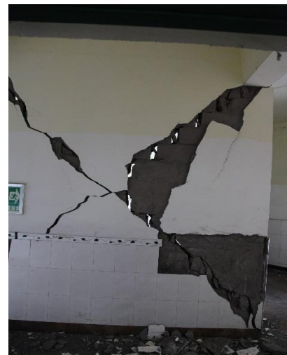
Fig.25 – Damaged masonry infill at the edge (principal) of the building
